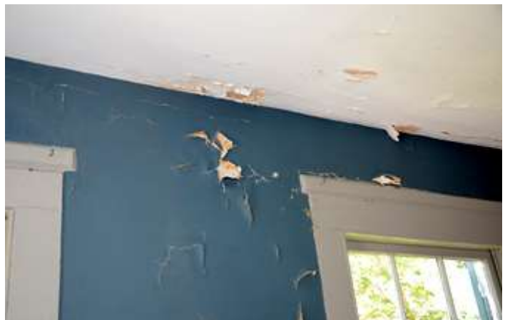
Peeling walls before preparation and re-paint
