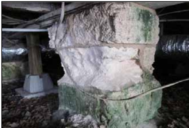
The old decaying limestone piers supporting the house were replaced with new concrete piers.
