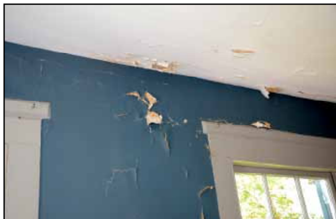
Peeling walls before preparation and re-paint.
